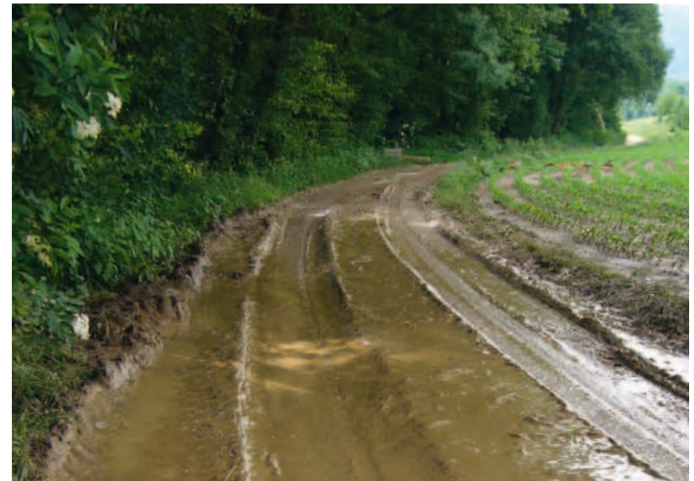
Eroded earth on agricultural track
